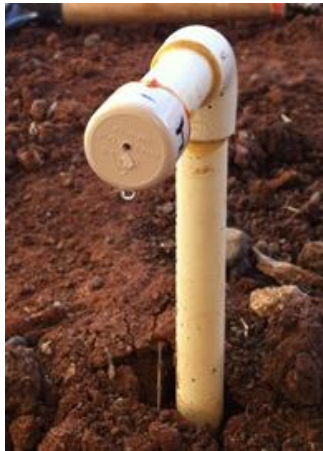
Figure 6. Irrigation system outlet pipeline.
